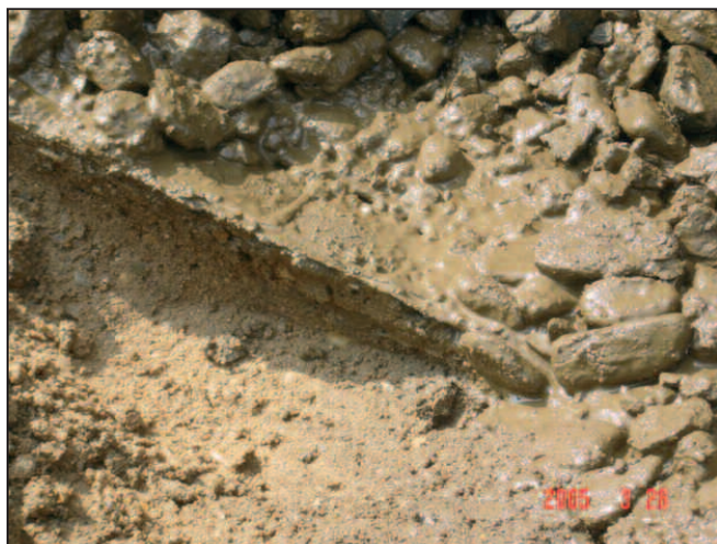
Fig. 1: Wet spot in the ballast bed
