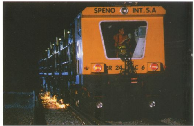
Fig. 3: The Speno RR 24 MC multi-purpose grinding train was used in a pilot project, aimed at developing new ways of working in awkward conditions (e.g. on bridges, and in switches and level crossings)
